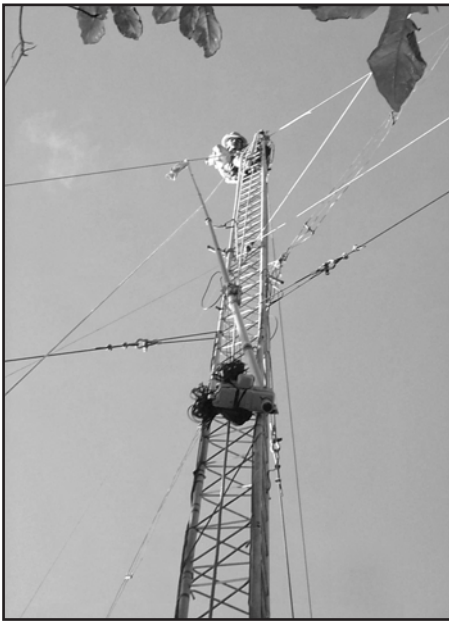
One of two SteppIR BiggIR verticals donated by NCDXF is hauled up the tower. Its tip is about 100 feet high, making it one of the tallest things on the island.
