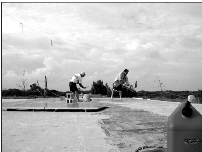
While on Kure, we had chores to do. Here, two team members paint the roof on one of the few remaining buildings.
