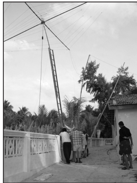
The Kadmat CW site where necessity is the mother of invention. Here a ladder had to be used instead of the unsuitable bamboo poles.
